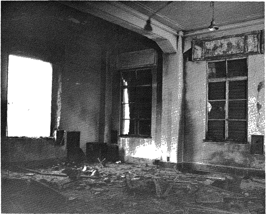
Figure 7.70. Fire shutters in building blown in or damaged by the blast; shutter at center probably blown outward by blast passing through building (0.57 mile from ground zero at Hiroshima).
